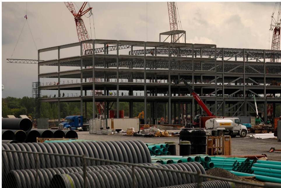
Construction is underway on a massive Amazon warehouse and distribution center in the Town of Clay, just outside of Syracuse, Thursday, July 23, 2020. It's identical to the project proposed for Grand Island.
