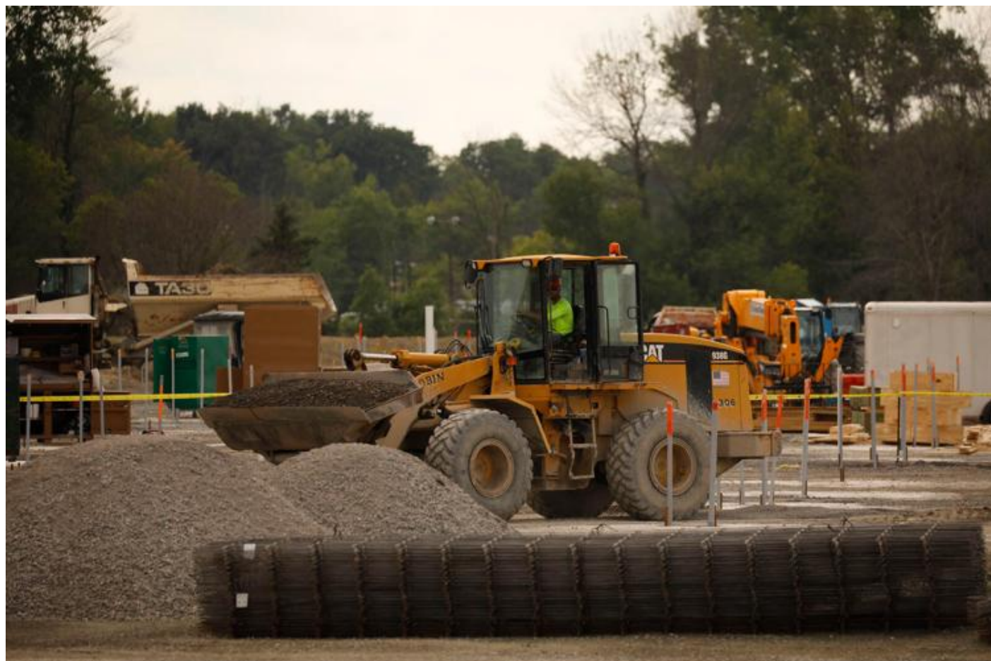
A bulldozer moves material around the massive Amazon construction site in Liverpool, just outside of Syracuse, Thursday, July 23, 2020.
