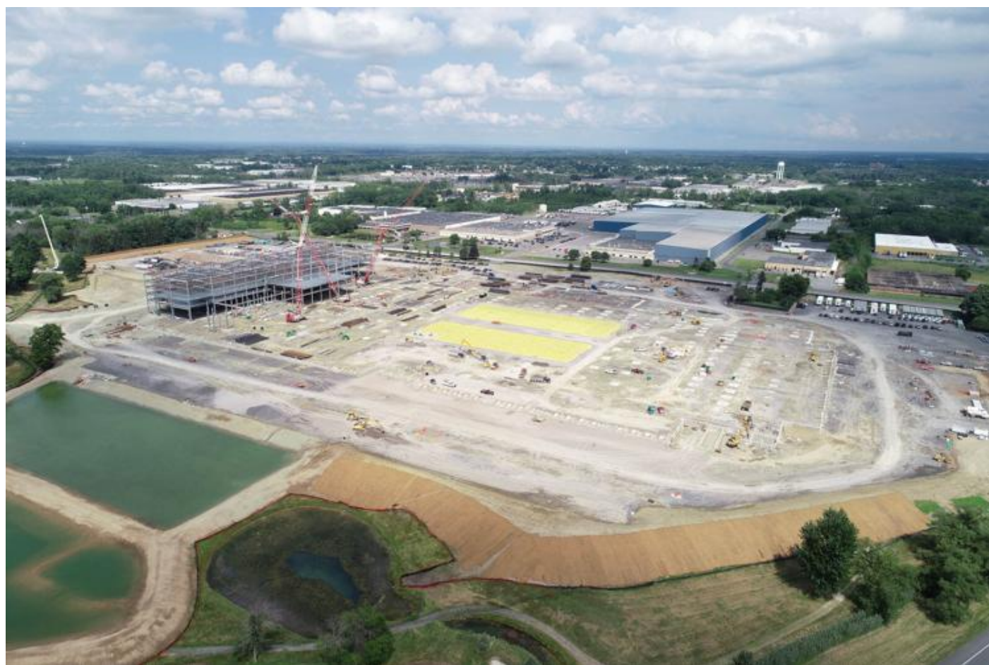
An aerial view of the massive Amazon site under construction on a former golf course in Liverpool, just outside of Syracuse, Thursday, July 23, 2020.
